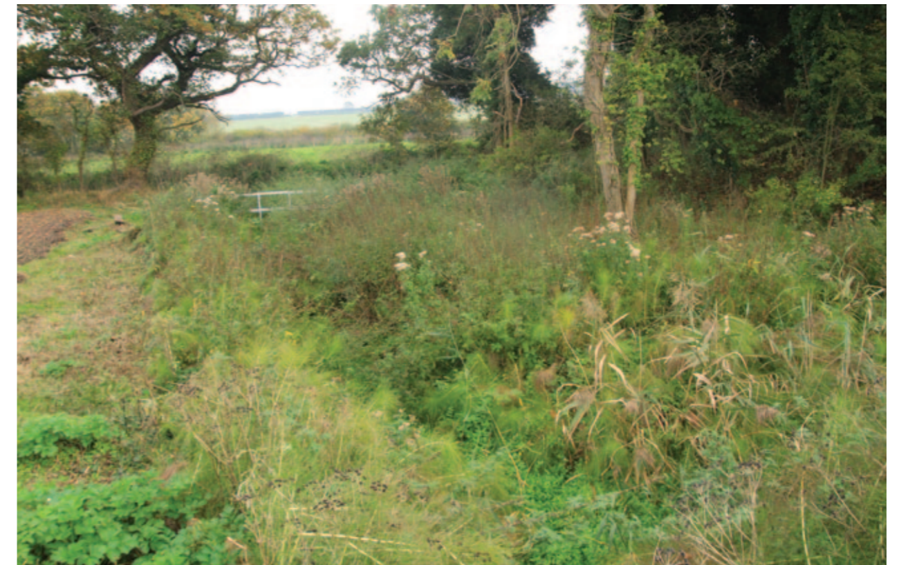
The old moat to the west of Holt Road is currently overgrown and full of silt.
